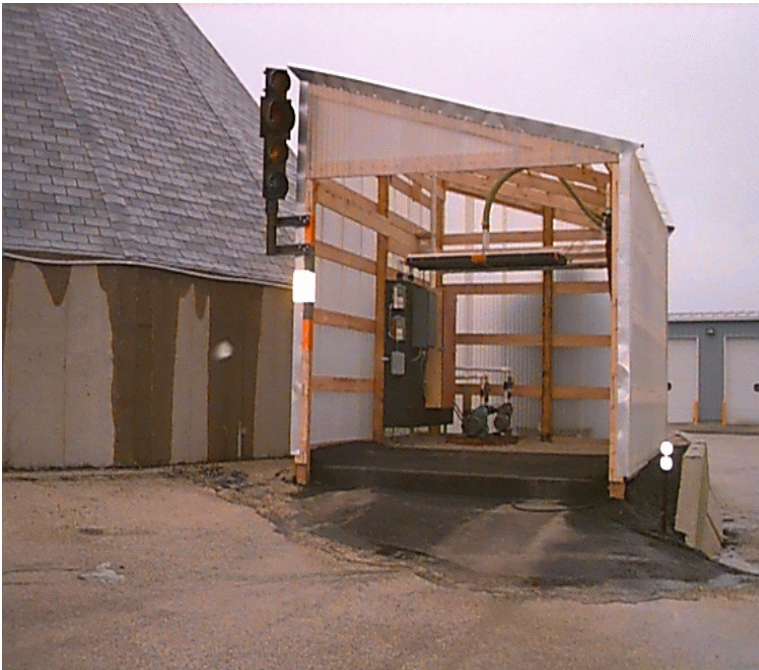
Figure 3: Prewet unit setup for prewetting an entire truck load at a time.
