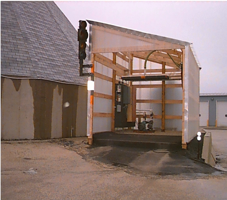
Figure 3: Prewet unit setup for prewetting an entire truck load at a time.
