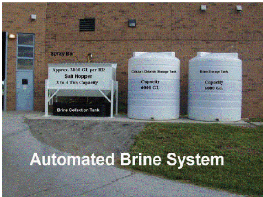
Figure 12-2 Automated brine system (mixing hopper and 2 – 6,000 gallon holding tanks)
